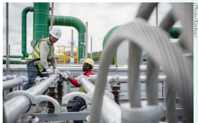
Construction crews work at the construction site of the Sosian Geothermal Power Plant project on May 26, 2023 in Nakuru, Kenya.
